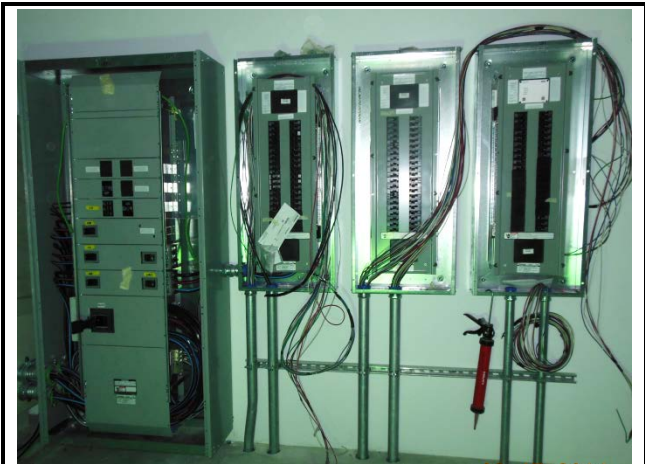
Service disconnect gear (left) and panels in Electrical Rm
